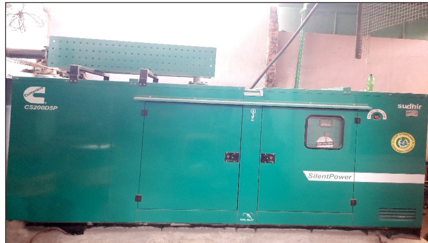
CUMMINS CS200 DSP 200KVA GENSET (NOS 01)
